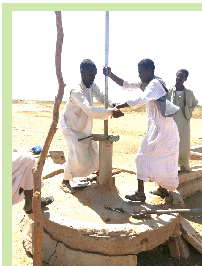
Returnee community from Darrasta repairing hand pump after receiving tools and training from Aqua4Sudan
